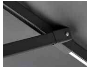
Brace joints and LED light strip
